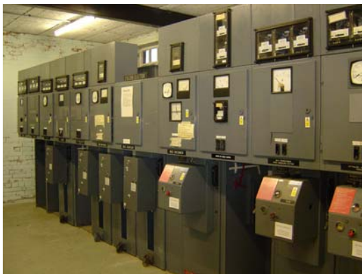
Picture showing partially retrofitted English Electric OLX Switchboard
